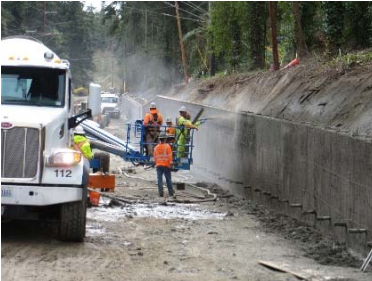
Three layers of concrete were applied to the wall and it was completed March 27th.
